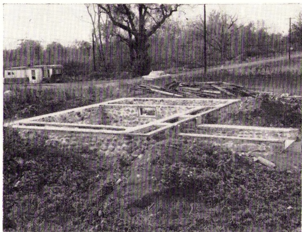
Another view of the cottage cellar showing the front walk foundation in place.
